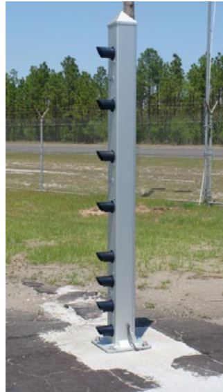
ACM 4/2 Anti-Climb Mast Installation (2meter tall)
